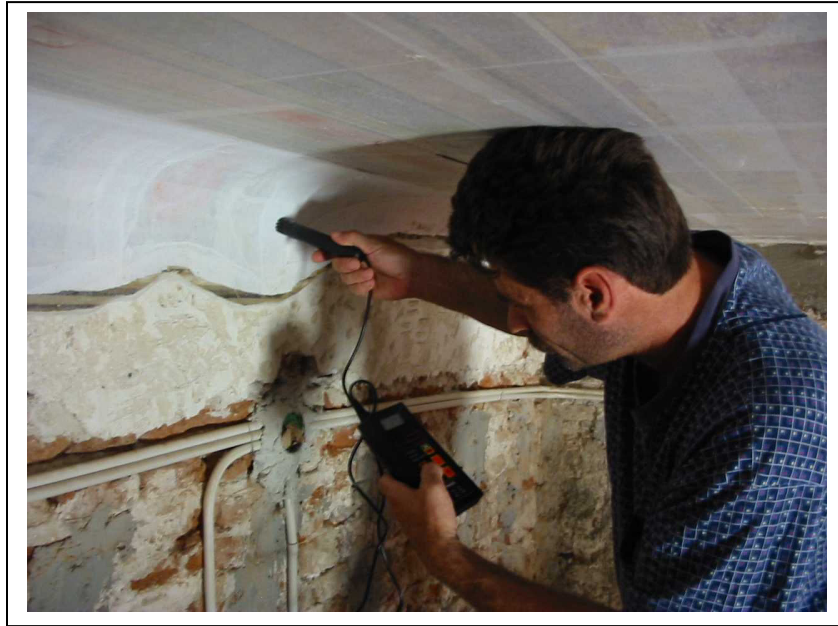
Figure 1. The monitoring of humidity and temperature.
