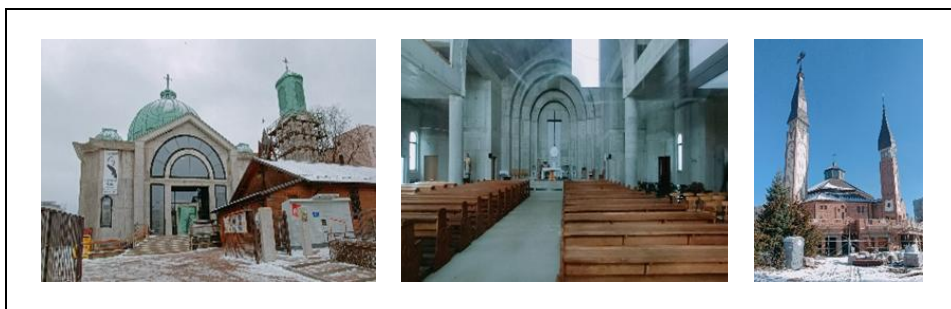
Figure 10. Examples of churches under construction in the Archdiocese of Lublin. Church and presbytery under construction - the Parish Church of Blessed Bishop Władysław Goral and the Parish Church of Biskupa Władysław Goral and the Transfiguration of the Lord in Lublin. Photograph by the author.
